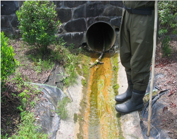
Storm drainage pipes often discharge pollutants, such as bacteria, fertilizers, and everyday household chemicals into local waterways.
